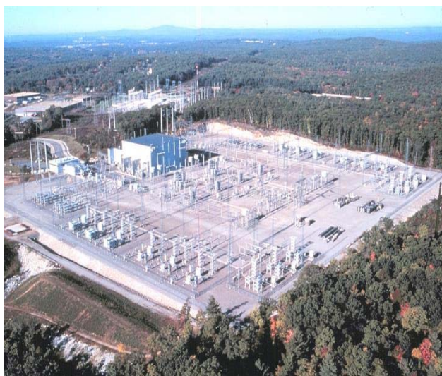
Typical 500 kV DC Converter Station
