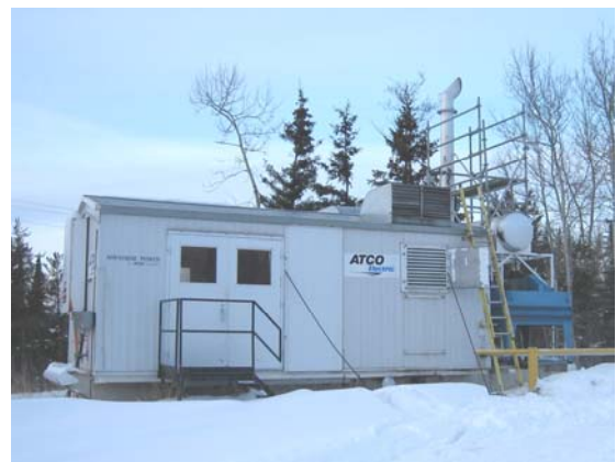
Typical Back-up Generator
