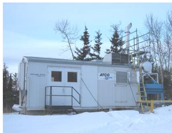
Typical Back-up Generator
