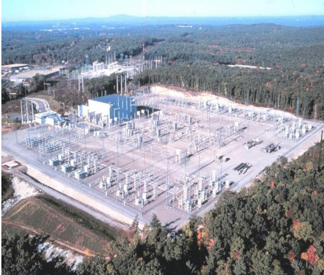
Typical 500 kV DC Converter Station
