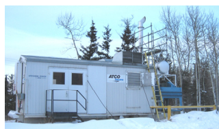
Typical Back-up Generator
