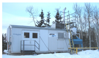
Typical Back-up Generator
