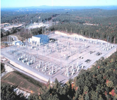
Typical 500 kV DC Converter Station
